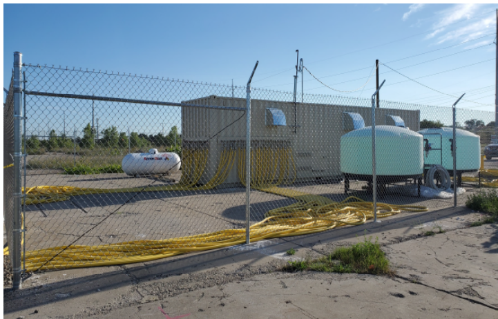
Plant 2 Biosparge Unit and Nutrient Injection Tanks
