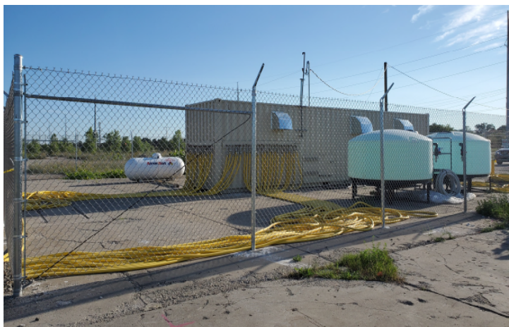
Plant 2 Biosparging Building, Propane Tank, Hoses, and Nutrient Injection Tanks
