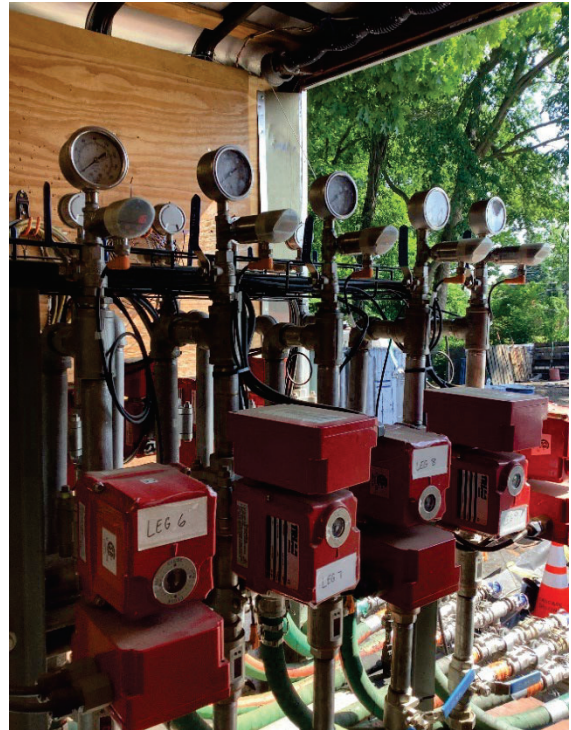
Photo G.13 Pathfinder Pumps and Pressure Gauges
