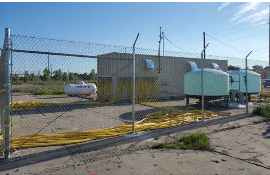
Plant 2 Biosparge Unit and Nutrient Injection Tanks
