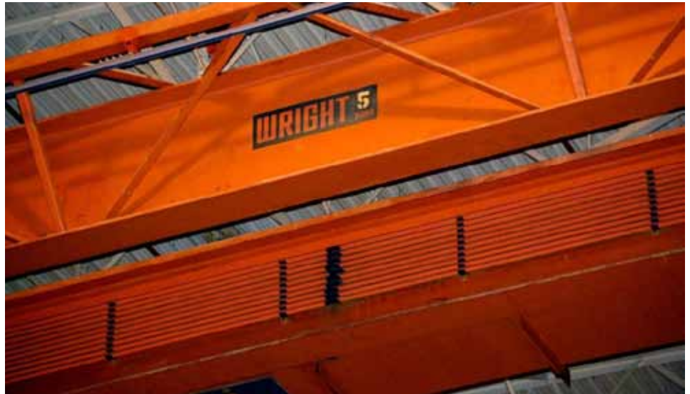
The manufacturing area includes a 5-ton overhead crane, seen here.
